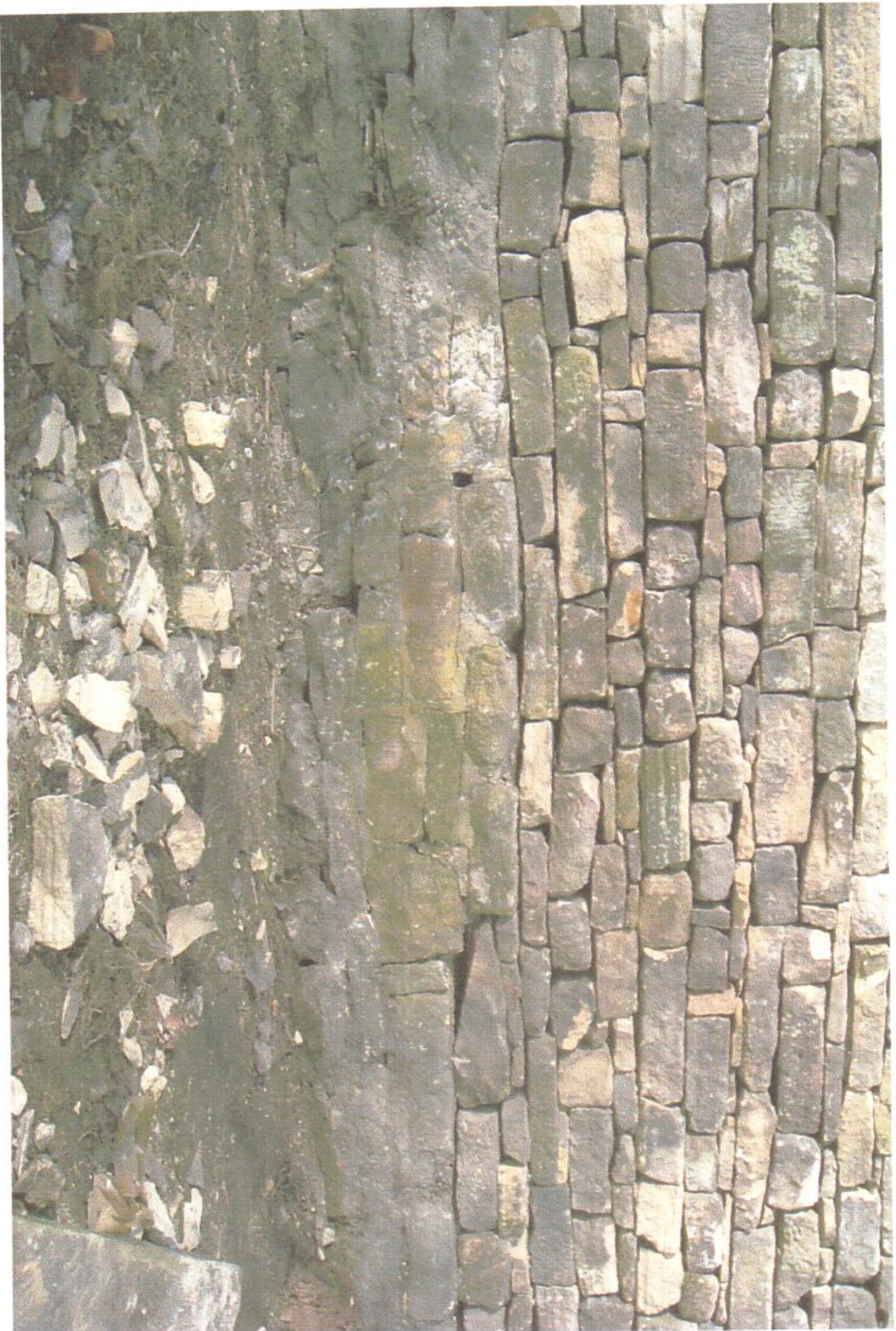
Figure 4. Stonework in the area to the rear of the Fox on top of which 18 th Century cottages were constructed. The new stonework on top is part of the construction of the new beer garden. The lowest courses have characteristics from several hundred years before the current building. Could these stones be the foundations of Margery's Tiddlewink?
